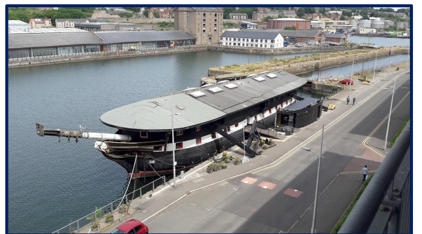
Roof Extension (Before & After) – The new roof at the front of the ship extends over the forecastle or foc'sle
